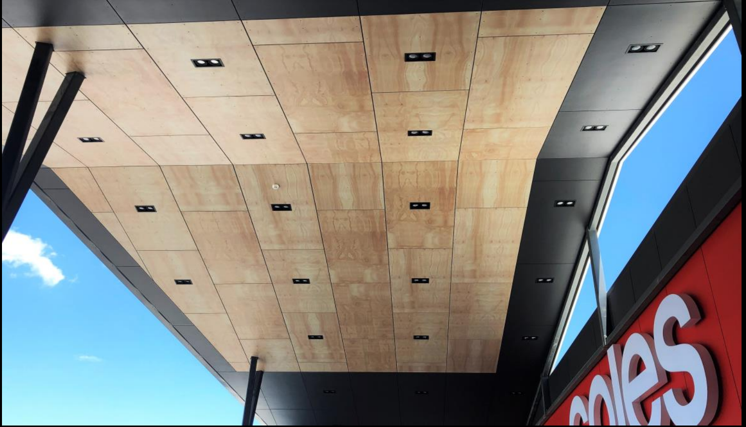
Karalee Shopping Centre—QLD Builder: Hutchinson Builders Product: Hoop Pine digital print on CFC panels
