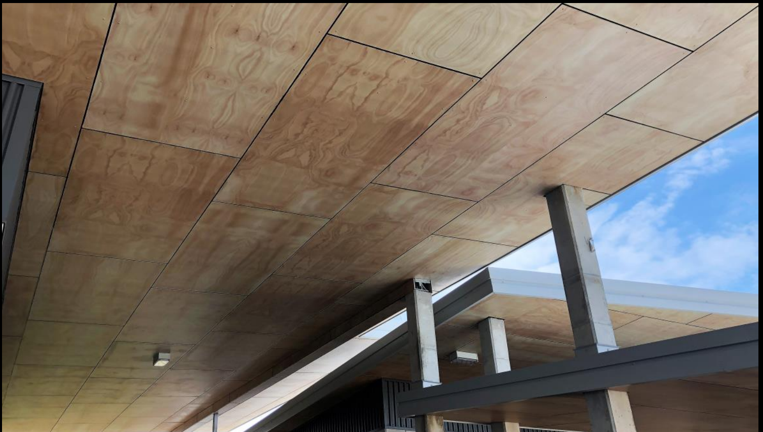
Pottsville High School—NSW Architect: Conrad & Gargett Installer: Ideal Commercial Linings Product: Digitally printed CFC panels
